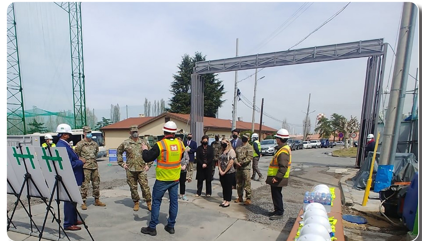
U.S. Army Corps of Engineers, Far East District Southern Resident Engineer, Jared McCormick, provided a tour and brief to the Army Family Tower #3 construction project at Camp Walker to Eighth Army-Korea Commander, Lt. Gen. Willard M. Burleson III, USAG Daegu Commander, Col. Edward Ballaco, USAG Daegu Command Sgt. Maj. Jonathan Blue, and their spouses on March 24. The project includes tower amenities like dog parks, picnic shelters, and bus shelters. Our team of engineers are dedicated to providing USAG Daegu the best facilities to take care of our community and to support the defense of the Republic of Korea. (Courtesy photo)
