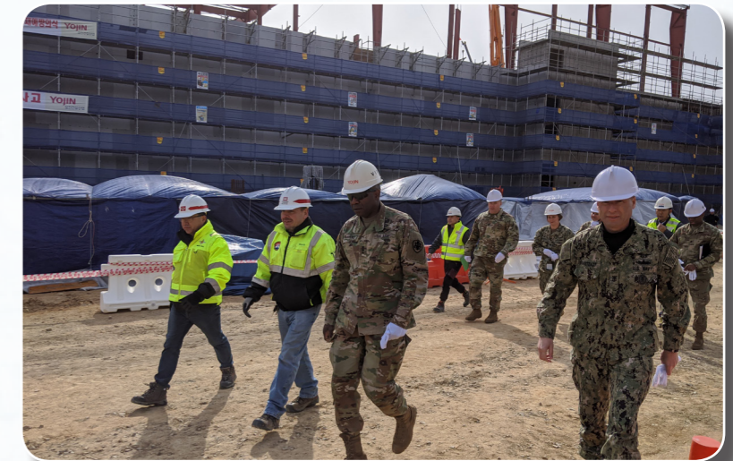
Lt. Gen. Darrell K. Williams, Director of the Defense Logistics Agency (DLA), paid a visit to the new DLA warehouse site to survey the current construction on Feb. 6 at Camp Carroll, South Korea. The warehouse will include a 20,000-square foot HAZMAT warehouse, 50 new parking spaces, and a three story administration office building. Fabio J. Vallejo, Quality Assurance Representative, Southern Resident Office briefed the director on the latest construction efforts. (FED file photos)
