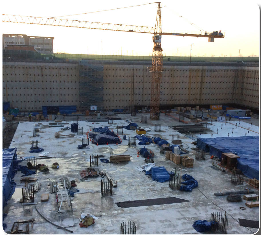
An overview of the construction progress on the United States Forces Korea Operations building set to be completed in 2020. (FED file photo)
