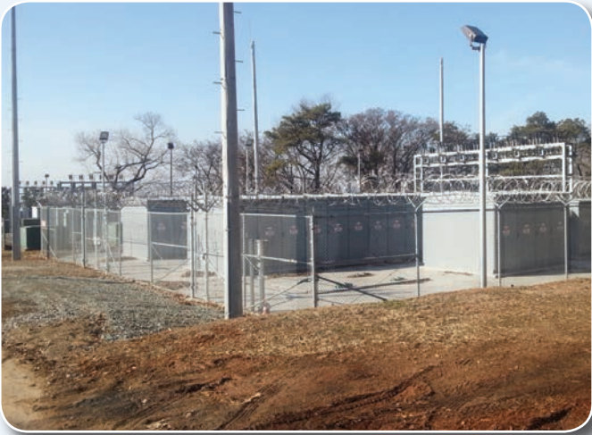
New switchgear at Beacon Hill
