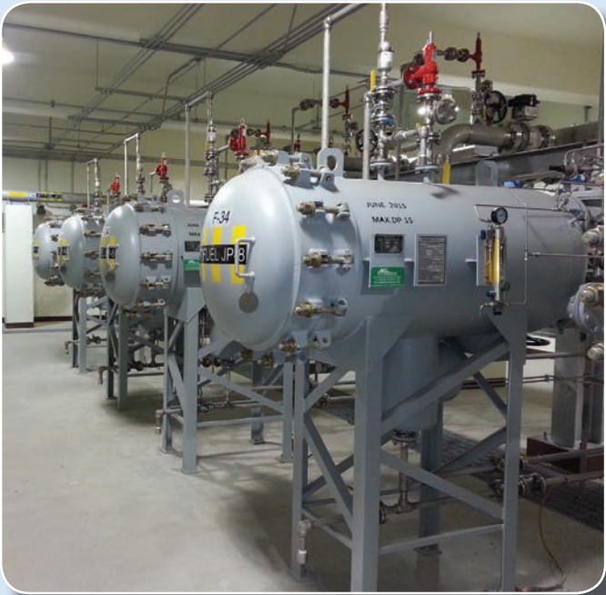
Hydrant Fuel System, Filter building
