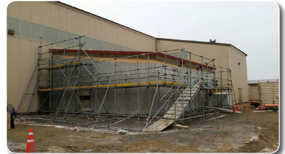
New Pump Room at Building 2241
