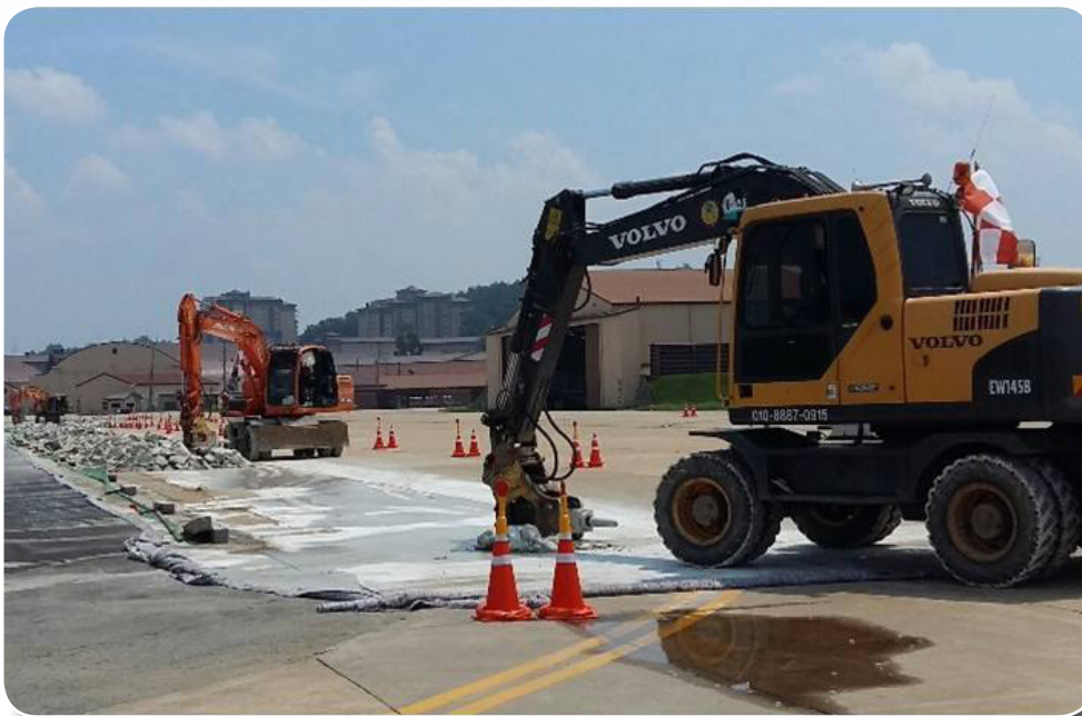
Far East District central resident office and Republic of Korea Ministry of National Defense-Defense Installation Agency finished repairs on the Osan Air Base Runway and construction on the southern portion of the new taxiway "C" Sept. 14. Taxiway "C" connects the new outside runway with the existing inside runway. (Photo by Frank Meleton)
