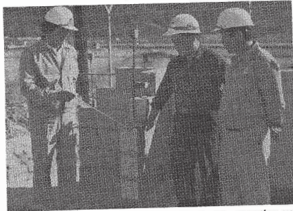
No, Hong Su, Project Manager for Daeho Construction explains their sample wall to O, Sung Sik (Western Corridor) as Daeho Quality Control Chief Yun, Chong Sung looks on.
