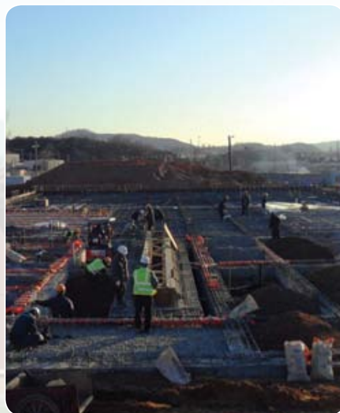
Construction is underway on a new barracks facility at U.S. Army Garrison Daegu. (Phot provided by FED Southern Resident Office)
