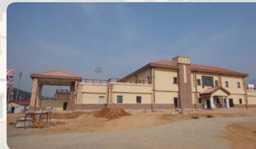
Almost completed, the U.S. Army Health and Dental Clinic at Camp Carroll is a long-awaited project at U.S. Army Garrison Daegu. (Photo provided by FED Southern Resident Office)
