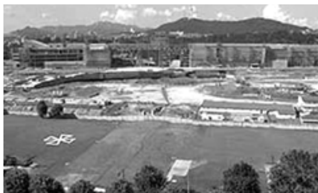
The USFK helicopter pad in Yongsan was located right next to the National Museum of Korea under construction.
