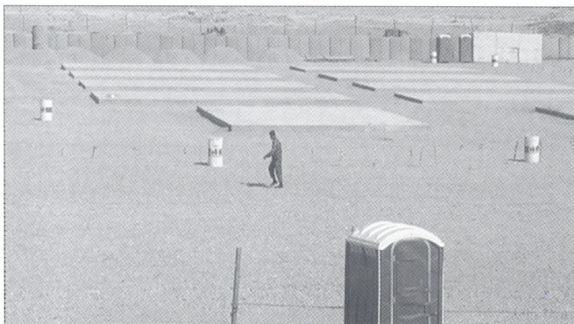
Pictured here are eight of the housing unit slabs and the two office unit slabs
