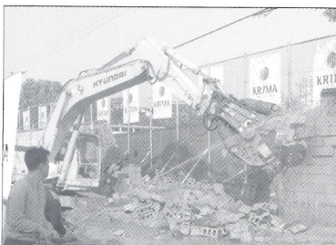
The wall between Yongsan Garrison and Ministry of National Defense is demolished in preparation for new helipad construction.
