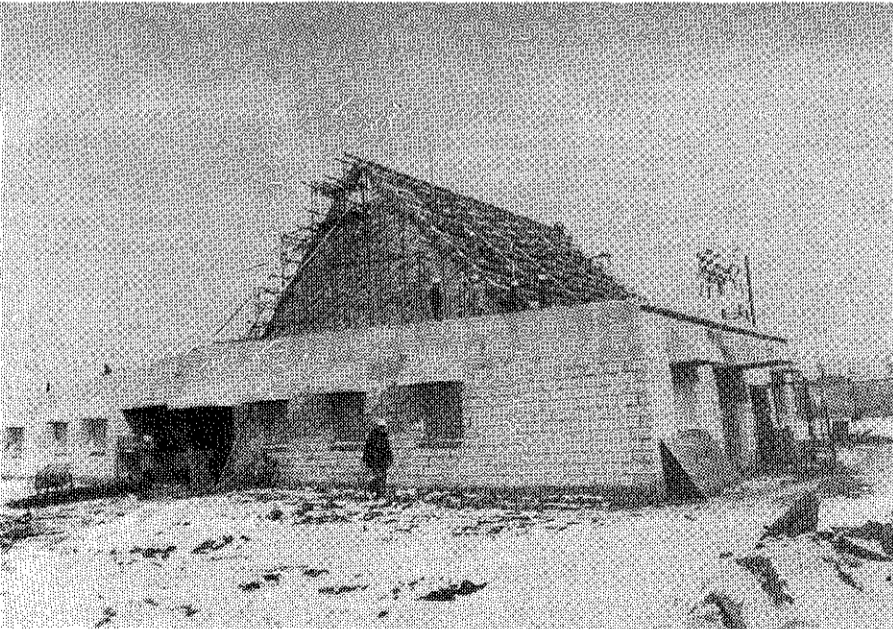
The Camp Humphreys Chapel is near 50% completion. The contractor is the Boo Hung Development Corporation.
